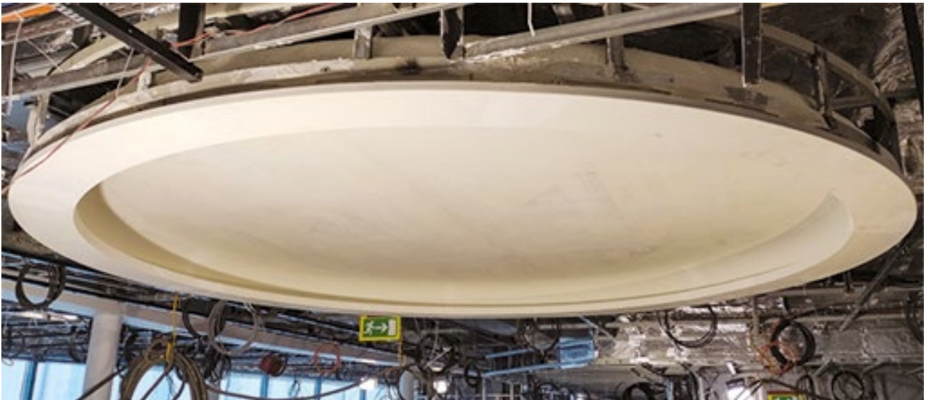
A layer of CA120 adhesive plaster, applied across the DGG sheet (short to short edge), levels any sheet surface rippling.
