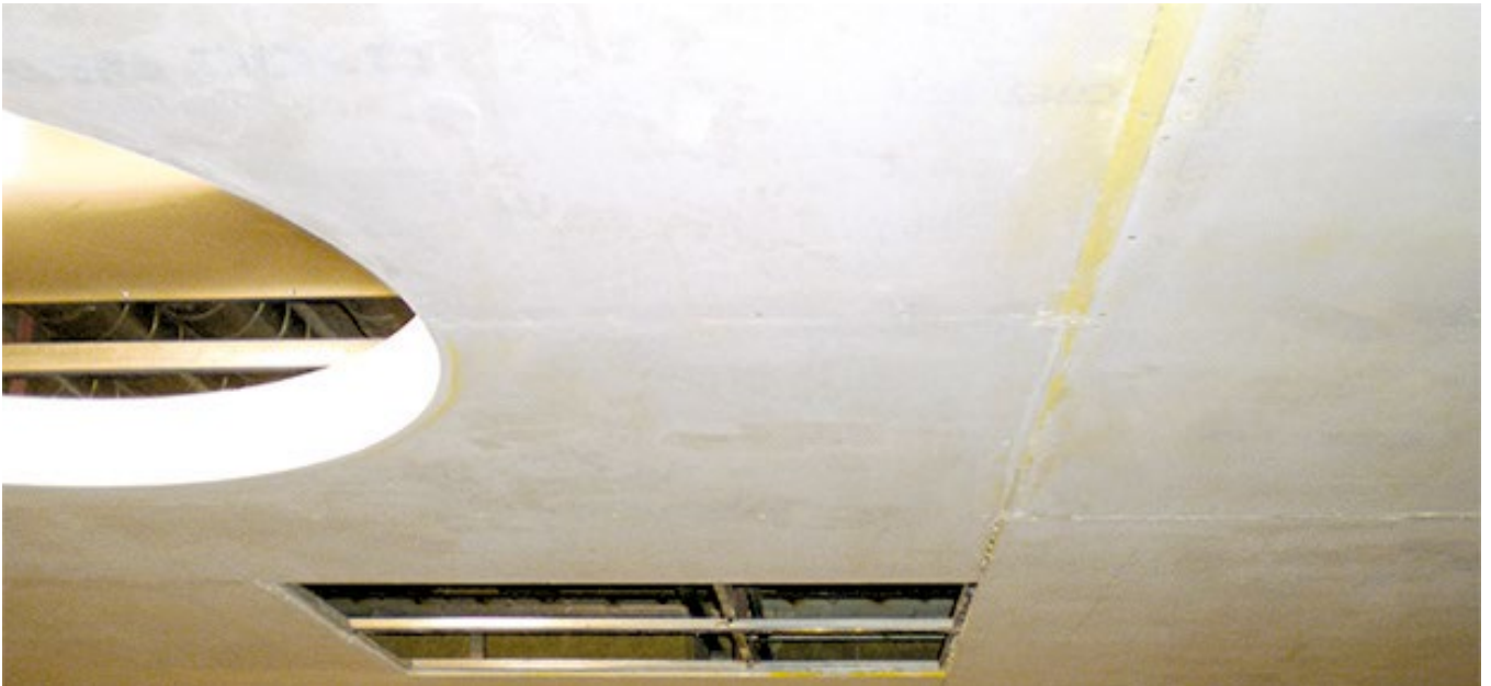
A layer of CA120 adhesive plaster has been applied across the DGG sheets. The yellow fiberglass mat is barely visible.
